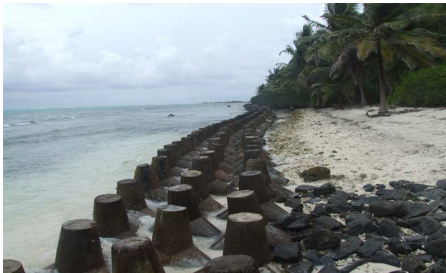
Seashore of Kalpeni Island protected with Tetrapole Seashore of Lakshadweep needs more protection measures under MGNREGA
